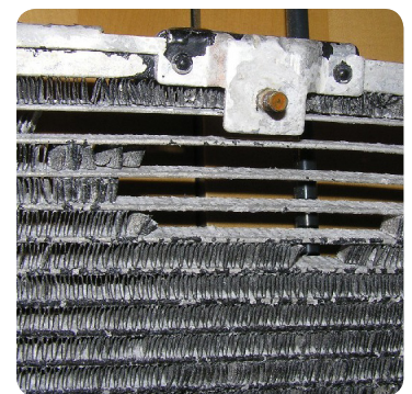
Several rows of missing fins caused by condenser corrosion
